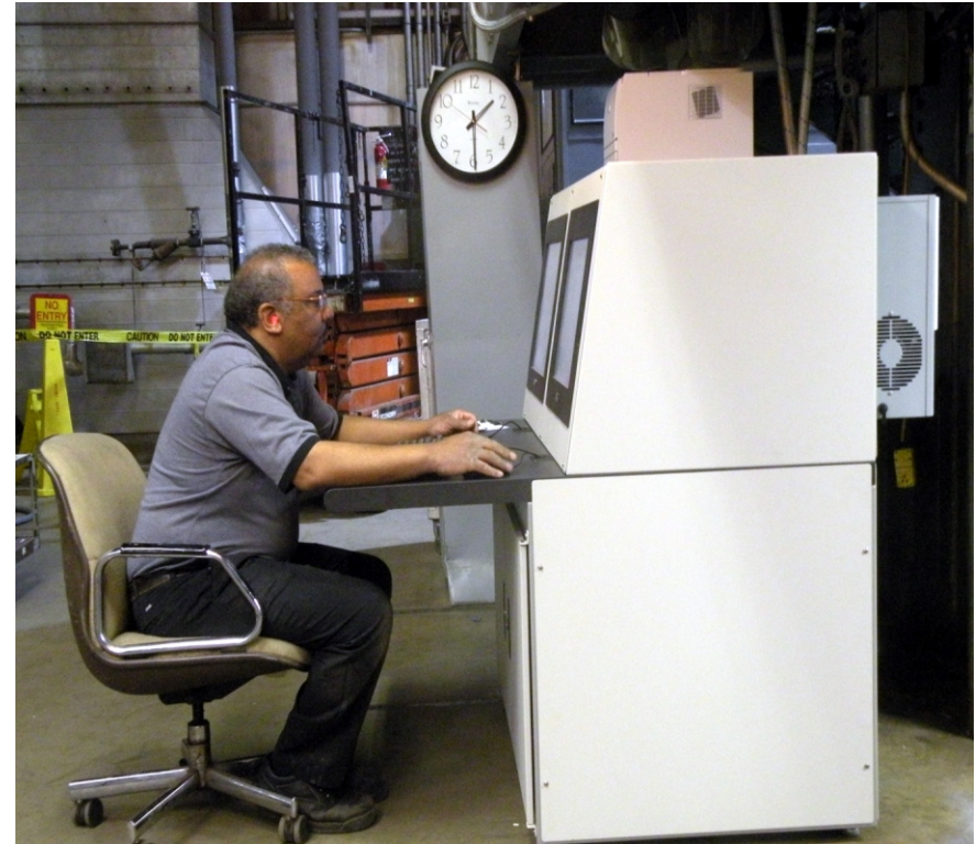
Customer field installed air conditioner Kooltronics Model KA4C2P28L - 2000 btu
