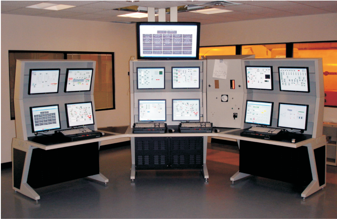
2-Tier Power Plant Operator Consoles with Privacy Panels - Note Cable Access at Back
